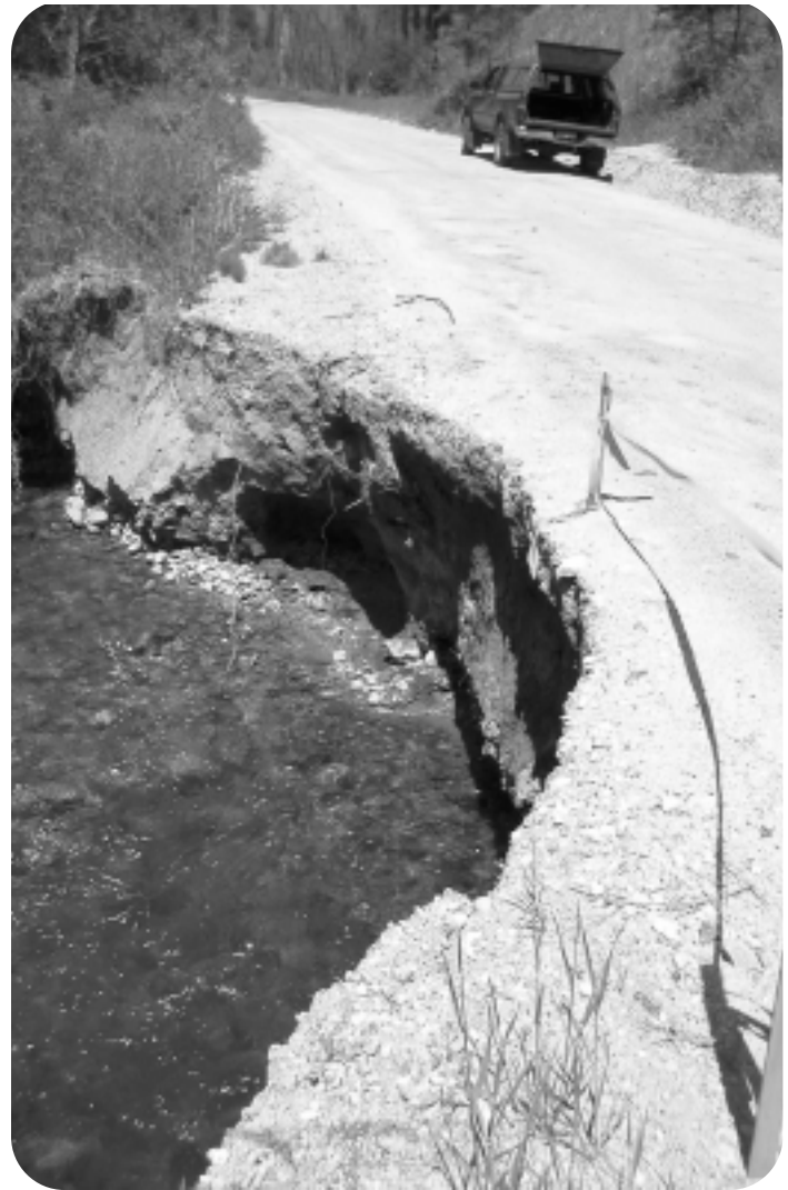
There are real, on-the-ground consequences associated with the Forest Service's failure to complete promised road and water restoration work as part of the "Burned Area Recovery Plan." With over $16 million slated for critical non-logging restoration and rehabilitation activities taken away from the Bitterroot Burned Area Recovery project by Chief Bosworth to pay for firefighting costs of the 2002 fire season, nearly 75% of the promised restoration work remains undone. Photo by Matthew Koehler.
