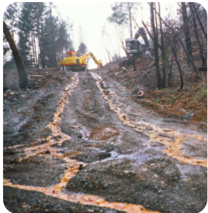
Heavy machinery causes erosion endangering high quality watersheds. Photo by Rolf Skar.
