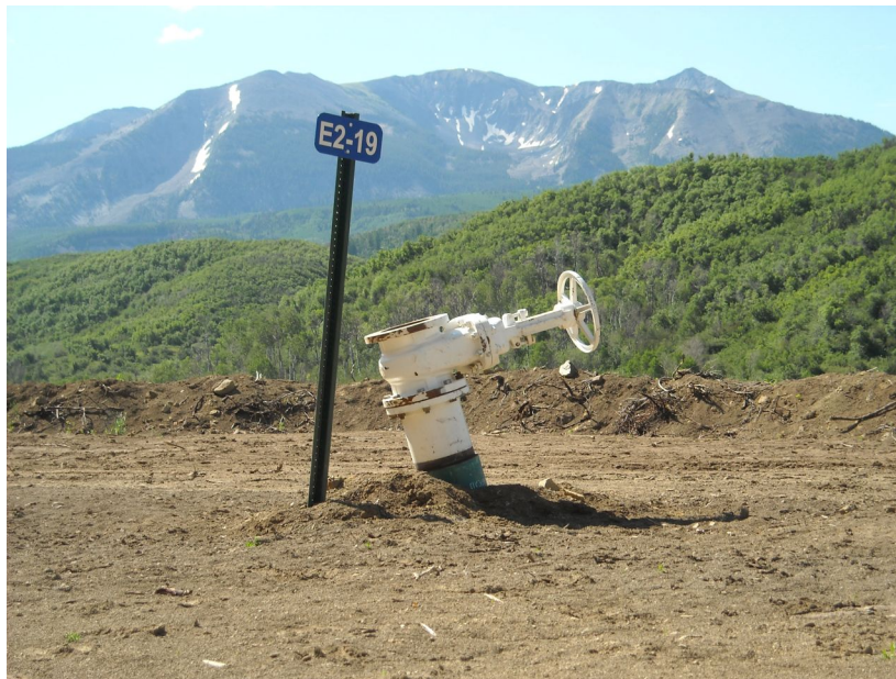
Methane venting well above West Elk Mine (view of Mount Gunnison in background). Picture taken June 30, 2010.
