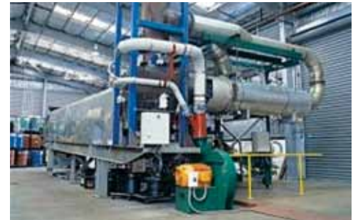
Hybrid waste coal/VAM rotary kiln (Photo courtesy of ComEnergy)
