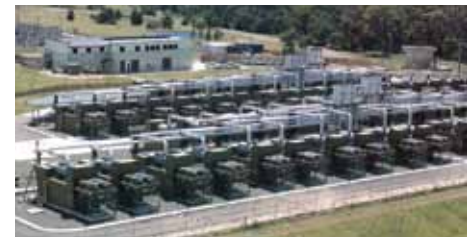
Appin power plant (Photo courtesy of EDL)
