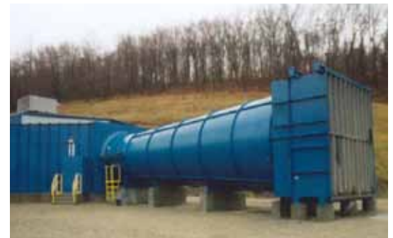
Ventilation exhaust (evasé) (Photo courtesy of H. Lee Schultz)
