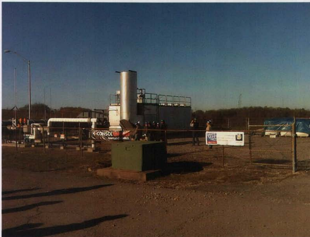
MEGTEC VOCSIDIZER system installed at CONSOL Energy's Windsor (closed) mine.
