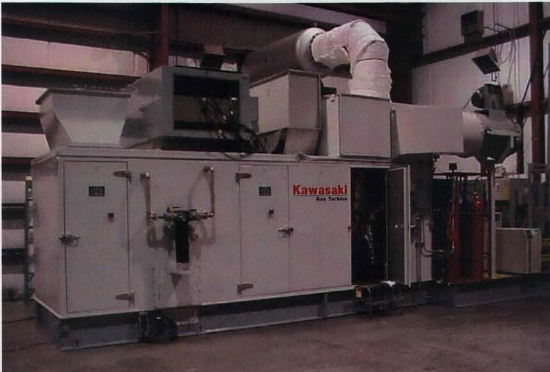
Figure 3-1: Kawasaki GPB15 Combustion Turbine
