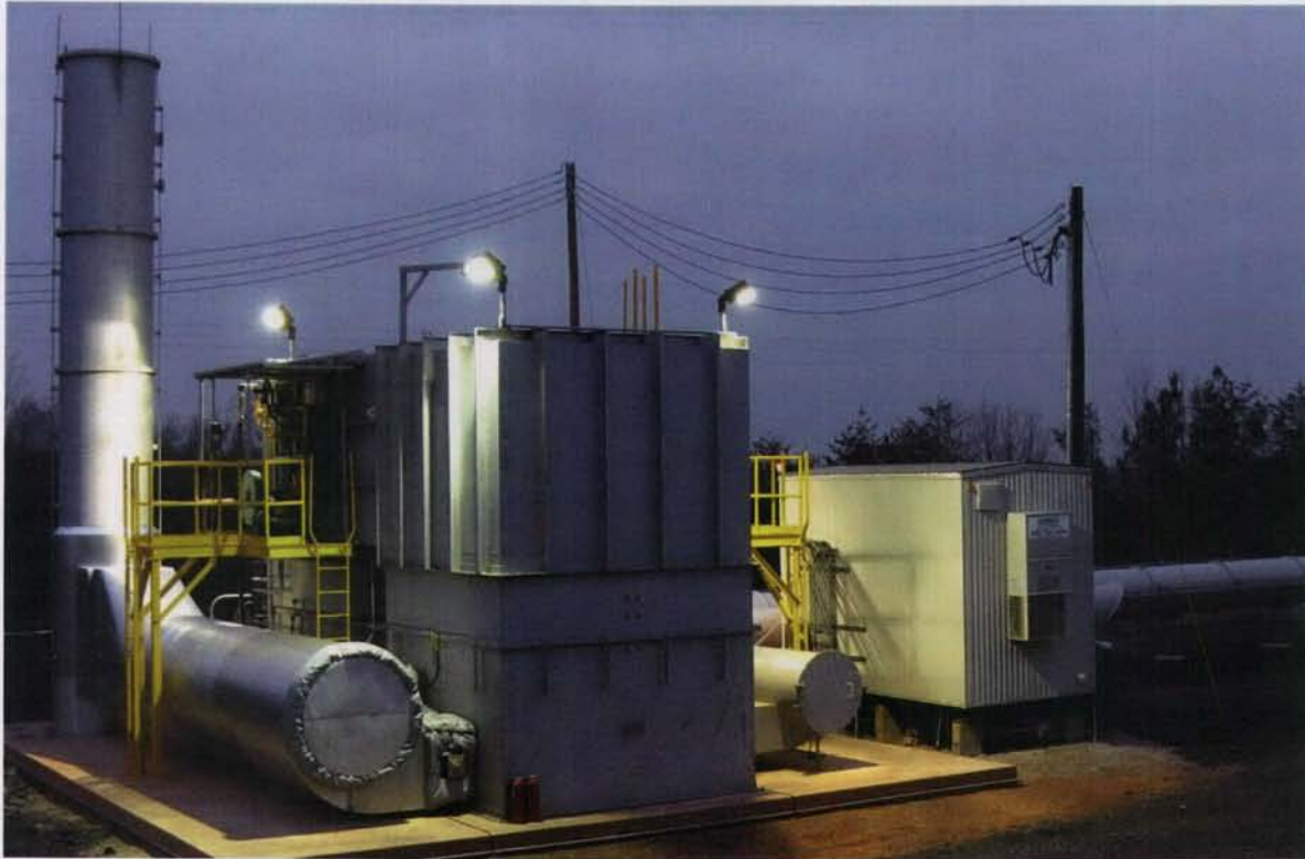
Biothermica VAMOX™ system installed at Jim Walter Resource's Mine No.4.
